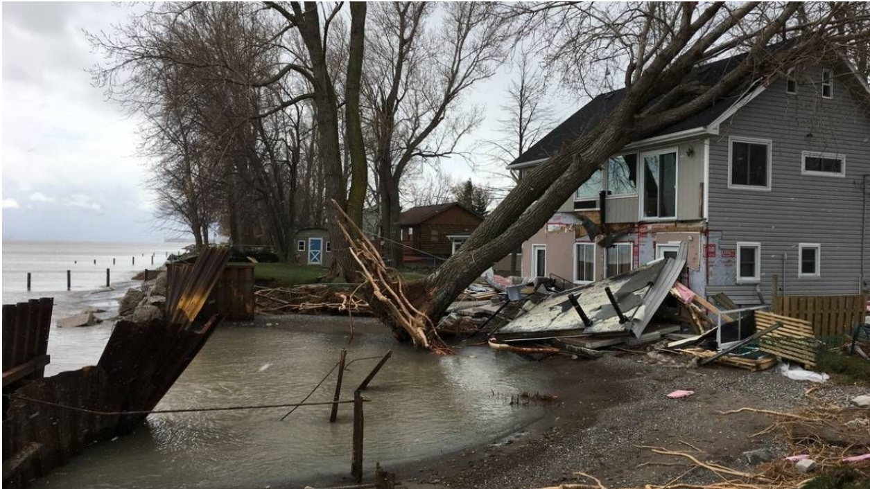
Figure 19: Failed seawall and home damage along Marentette Beach (south of HMCA) following the April 2018 ice storm.
