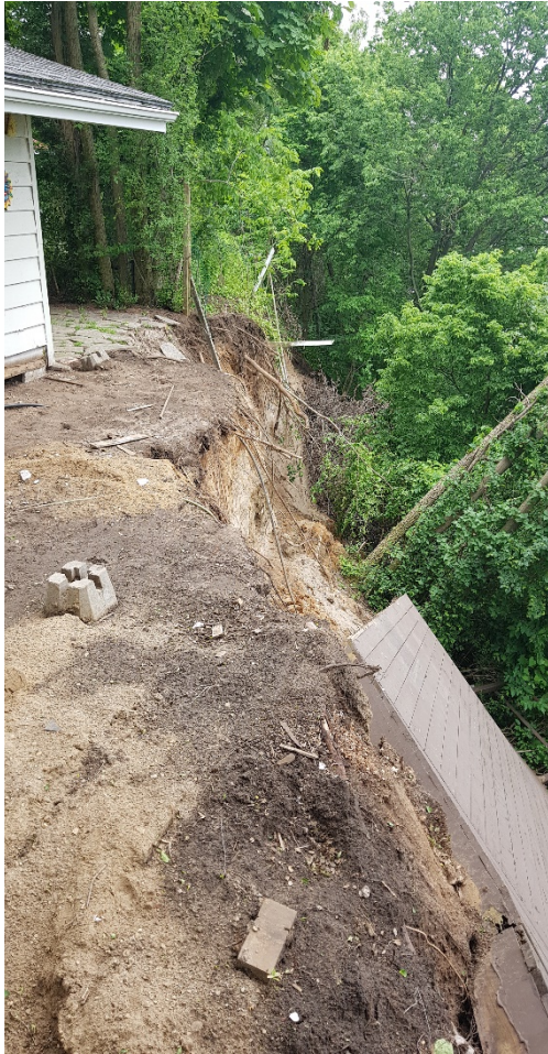
Colchester Bluff Failure
