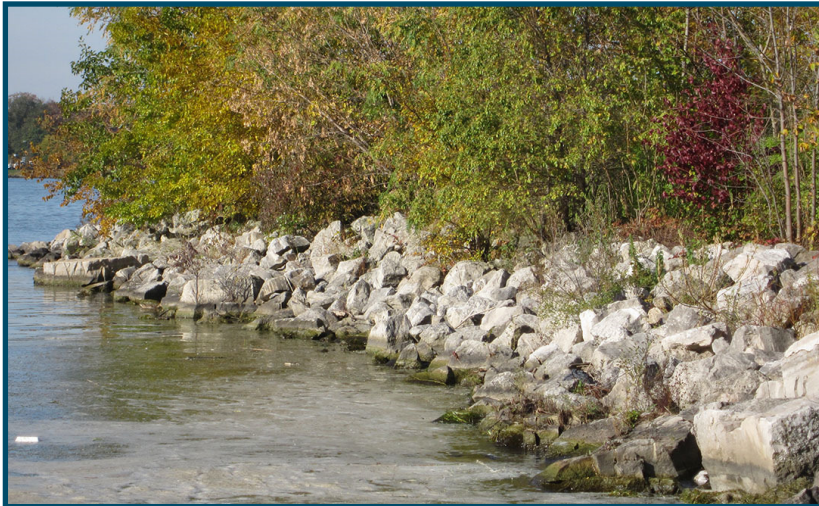
Vegetated Backshore along Goose Bay Revetment (between Jos Janisse Ave and Pillette Road)
