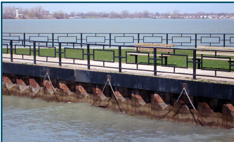
Steel Sheet Pile Breakwall at St. Rose Beach (at St, Rose Avenue)
