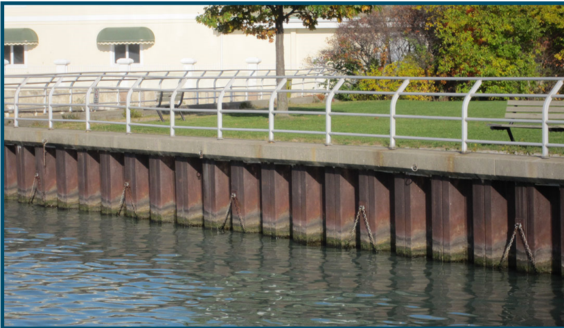
Steel Sheet Pile Wall East of St. Paul Pump Station (between Eastlawn Avenue and Lauzon Road)
