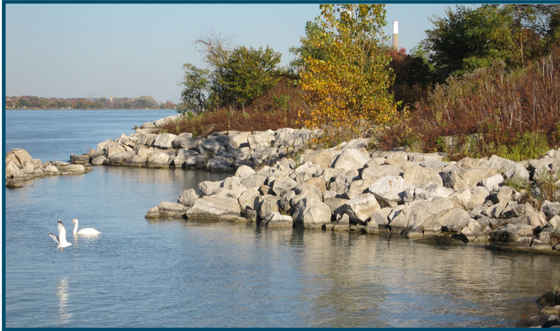
Hatch Gardens Armour Rock Revetment (between Langlois Avenue and Moy Avenue)
