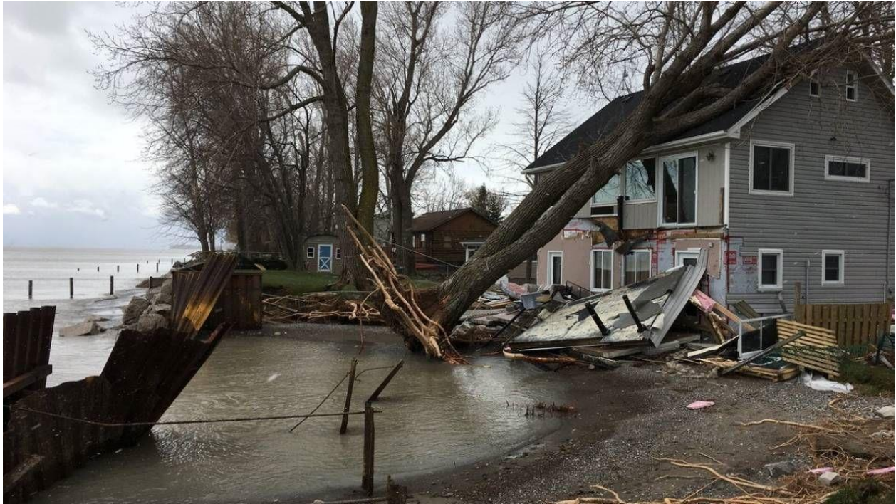
Figure 19: Failed seawall and home damage along Marentette Beach (south of HMCA) following the April 2018 ice storm.
